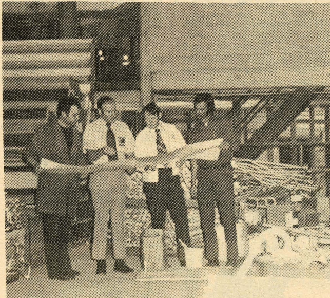
CHECKING RANGE BLUE PRINT - Tony Vaughan, second from left, Assistant Plant Engineer checks over new Polyurethane Range blueprint with engineering crew at installation site on the first floor of the Grier Division. Final increments of the Range, longer than a football field when finally erected, arrived at the Grier Division in late March. In photo above, left to right: Rovetti Arcangelo of Vicenza, Italy; Tony Vaughan; Jim Funderburk, RHP & F Draftsman and Bill Smith, Bleachery Mechanical Department.
