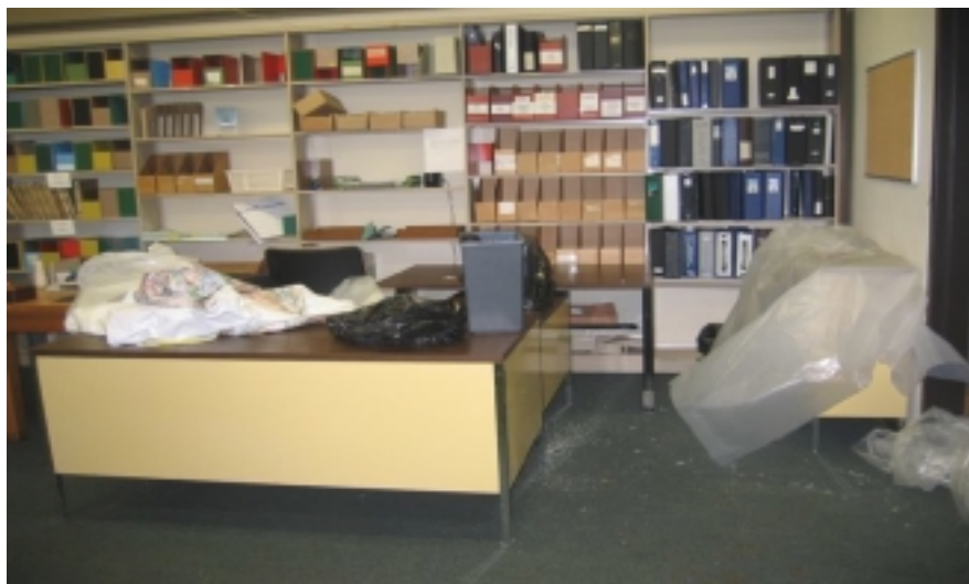
The Government Documents Office was flooded several times prior to the replacement of the roof.
